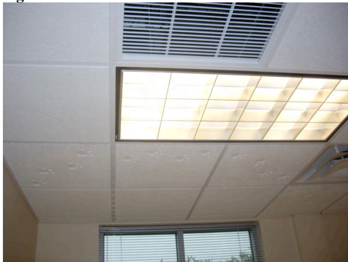
Figure 4.12: Ceiling Imprints throughout the Medical Ward
