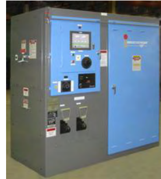
Figure 23. Induction Power Supply.
