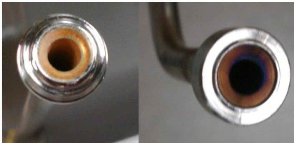
Figure 2.7: Contamination found in lines during system overhaul.
