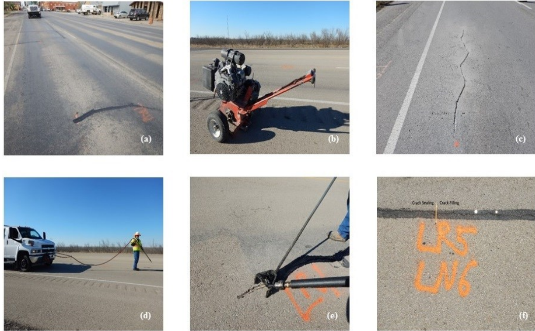
Figure 5-2. Crack treatment process (a) Longitudinal and transverse cracks; (b) Router; (c); Routing of cracks; (d) Cleaning of cracks; (e) Placing of sealant material with squeegee flush to the surface of the road; (f) Evaluation of the performance
