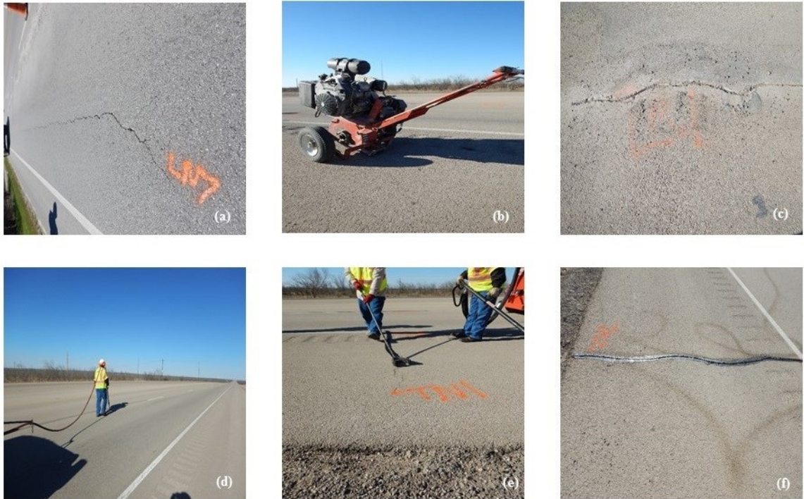
Figure 7-1. Crack filling and sealing process (a) Selection of cracks; (b) Router; (c); Routed crack; (d) Crack cleaning; (e) Sealant material installation with squeegee; (f) complete installation of crack treatment
