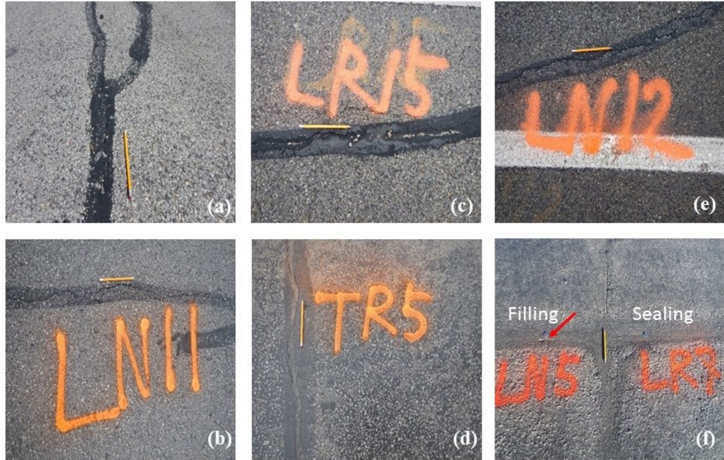
Figure 5-10. Visual assessment of crack treatment: (a) and (b) Loss of sealant material with filling treatment; (c) and (d) Adhesion failure of sealant material with sealing treatment; (e) Total failure observed with filling treatment for longitudinal crack; (f) Comparison between the two types of treatment
